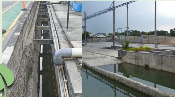
Installation of water management in each factory
