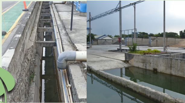
Installation of water management in each factory
