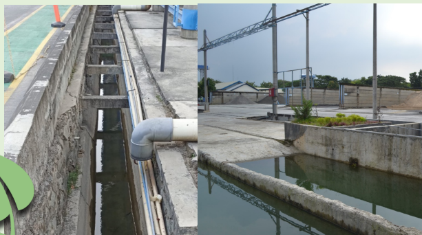
Installation of water management in each factory
